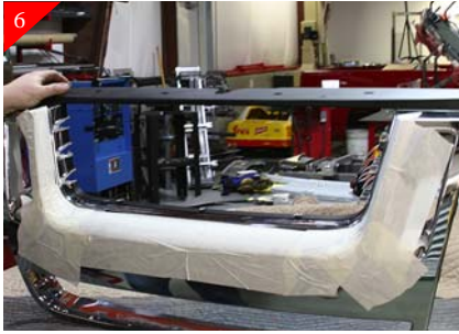
After center section is removed you will need to sand all cut areas smooth using a sanding block.
